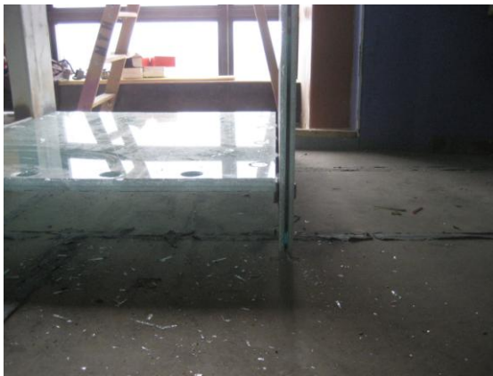
Figure 11: All Floor Panels Broken Retain Stiffness
